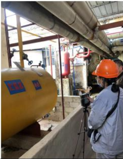
储氨罐 氨检测 2021-12-17
